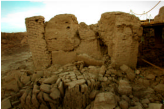
Figure 15: A massive pier composed of different periods and types of Khesht and chineh construction that have separated from each other during the earthquake.
