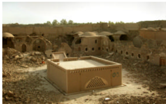
Figure 9&10: Before (November 2003) and After (April 2004) of the same view of the Stables courtyard showing the superstructure over the cistern that was recently reconstructed in fired bricks.
