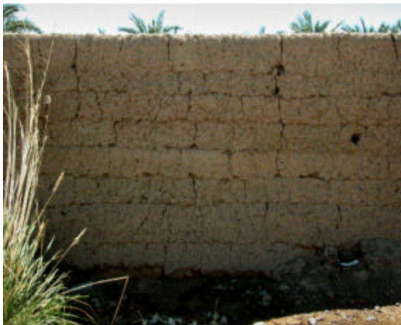
Figure 23: Chineh garden wall, probably of recent origin, in Baravat (near to Bam). This wall shows the cracks that commonly exist in chineh walls, and how the layered construction helps to ensure stability by allowing the cracked sections of the mud layers to perform like large blocks of masonry.
