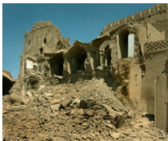
Figure 14: Buildings above the Stables courtyard that collapsed from the lateral spreading failure of the retaining wall and fill beneath.
