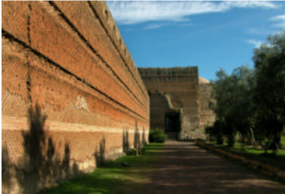
Figure 25: Long Wall, Hadrian's Villa near Rome showing the bands of brick that were laid into a wall constructed with natural cement with a tile facing. The crevices are the result of the later chipping out of the bricks for re-use.
