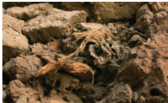
Figure 12: View of section of earthquake-caused collapse showing timber consumed by termites.
