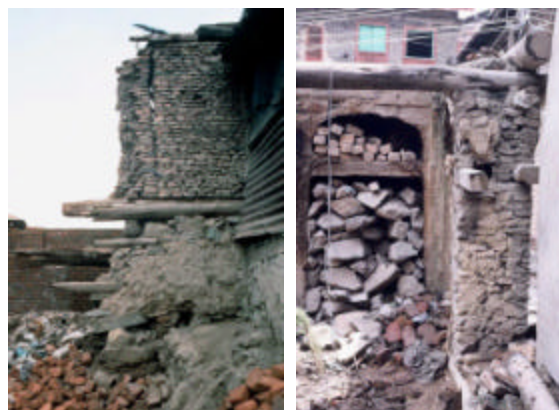
Figure 22: Two views of a multi-story dwelling under demolition in Srinagar, Kashmir showing the timber lacing laid horizontally into walls of masonry with mud mortar.
